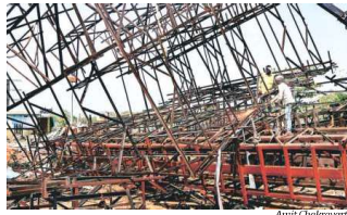
lars from the ground. Following that, mud was removed and samples of concrete at the base of the pillars were taken to VTI. The pillars were seen a few feet deep below which piling work was seen underground.
