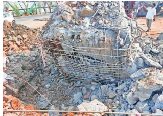
The base of one of the five pillars of the hoarding that collapsed. The depth of these pillars appears to be just a few feet below the ground; (below) oversized hoardings near the collapse site being dismantled.
